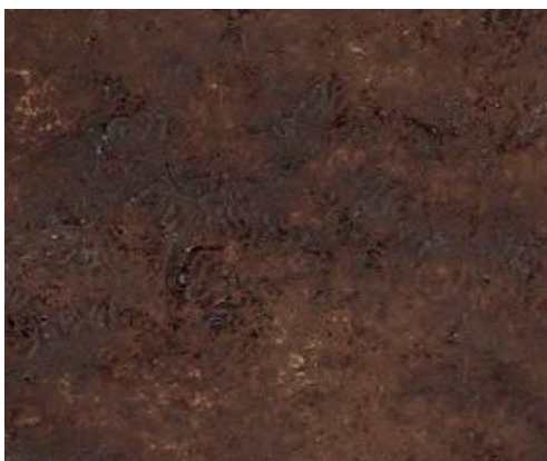
Metal rust - Red
