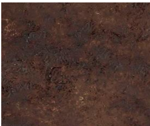
Metal rust - Red
