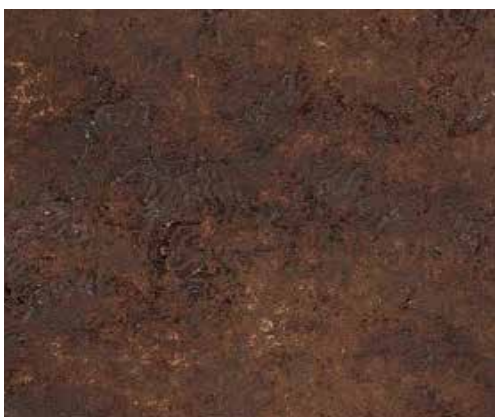
Metal rust - Red
